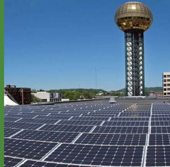
Solar panels on top of the Knoxville Convention Center
